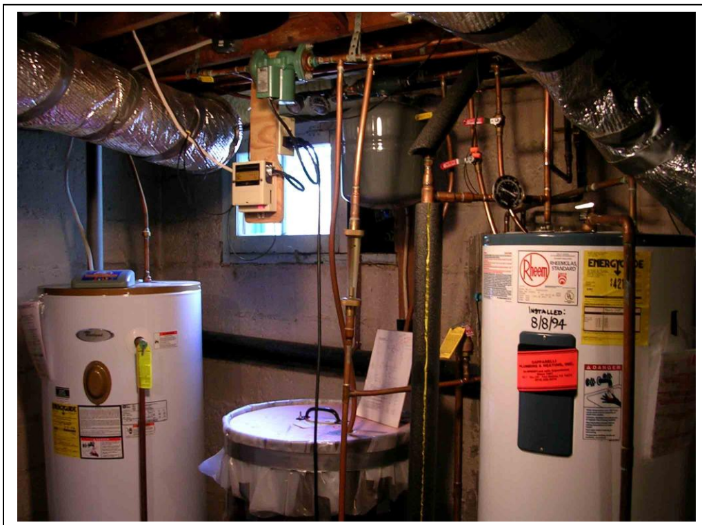
Above: Picture 6. Completed plumbing for our two tank pressurized glycol system
