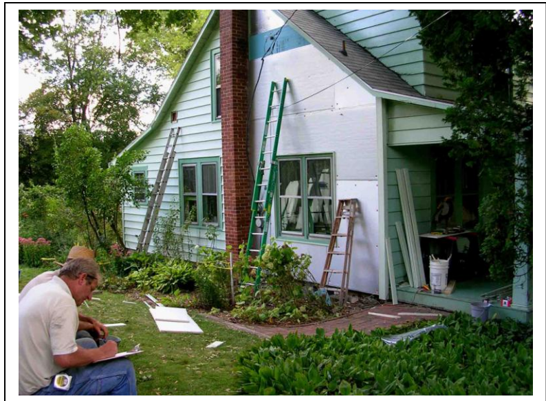
Right: Picture 1. East wall retrofit: adding two 1” layers of foamboard after removal of vinyl siding
