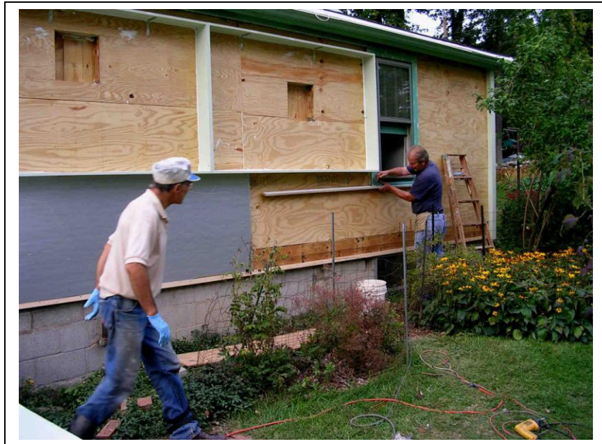
Above: Picture 5. Gene working with Howard Kephart, contractor. We nailed sheathing over foam-filled stud cavities, installed frames for hot air collectors, and are now nailing 1” foamboard. We will nail siding over this.
