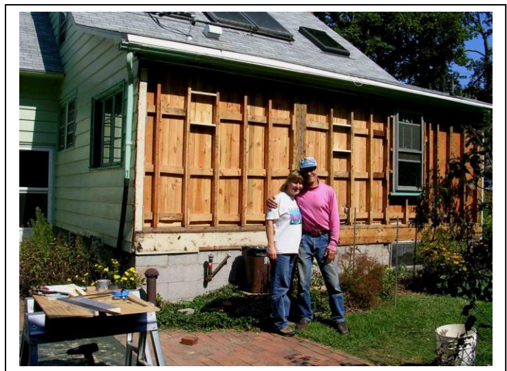
Right: Picture 3. South wall retrofit: Tania and Gene in front of wall cleaned down to studs, with holes for hot air collector vents framed
