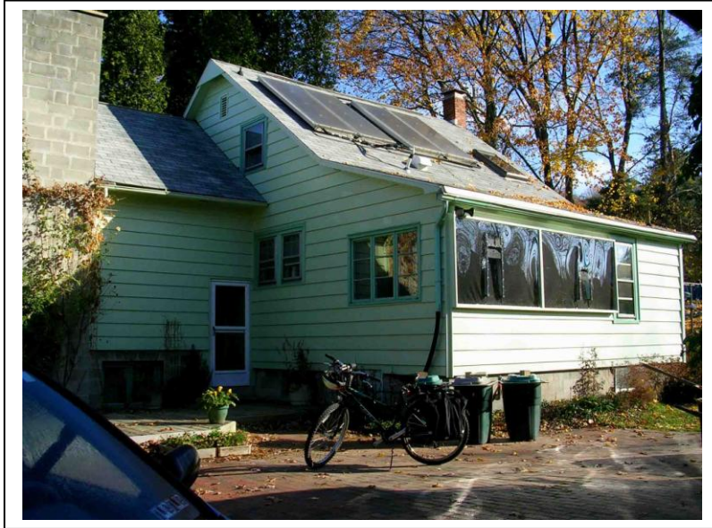
Left: Picture 8. Both collectors completed, absorbing heat
